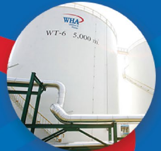
Utilities and Power
